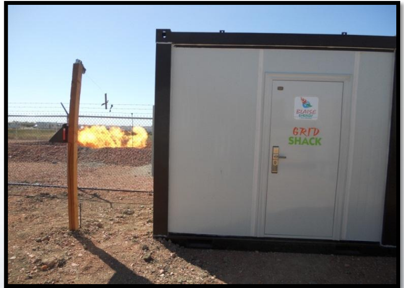
“Grid Shack” – All electronics & breakers to parallel to grid
