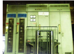
Thyristor Controls for Mud Pump
